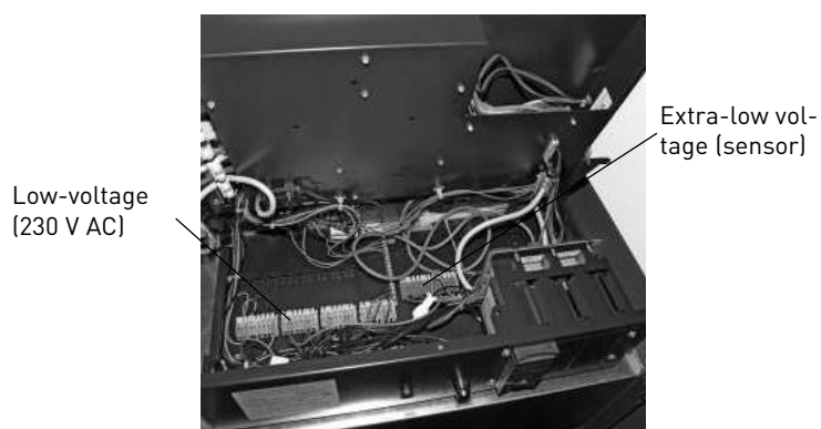
Fig. 87 Control panel bottom part with terminal blocks
